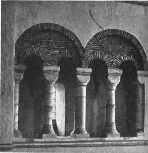
SAXON BALUSTER SHAFTS IN SOUTH TRANSEPT. (Photograph by Mr. W. H. Cox, St. Albans.)
